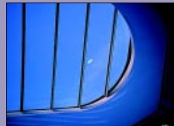
The rooflights above the stairs show a slight tendency towards air leakage.
