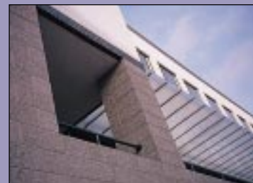
Some areas were initially underheated, like this first floor corner room above a walkway.
