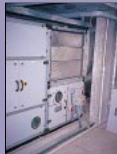
The heat recovery systems for two of EFry’s air handling units use high-efficiency heat exchangers. These are claimed to recover 85% of the available heat, a figure verified by the monitoring.
